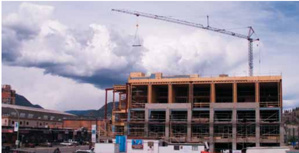
The Cannery Lofts, one of many multi-family developments under construction in 2004, is indicative of a trend towards greater interest in a more urban lifestyle.
