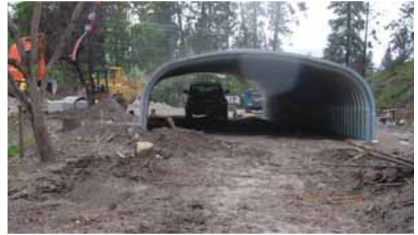
This Lebanon Creek culvert was the largest installed as part of $2 million in drainage upgrades after the 2003 Okanagan Mountain Park fire.
