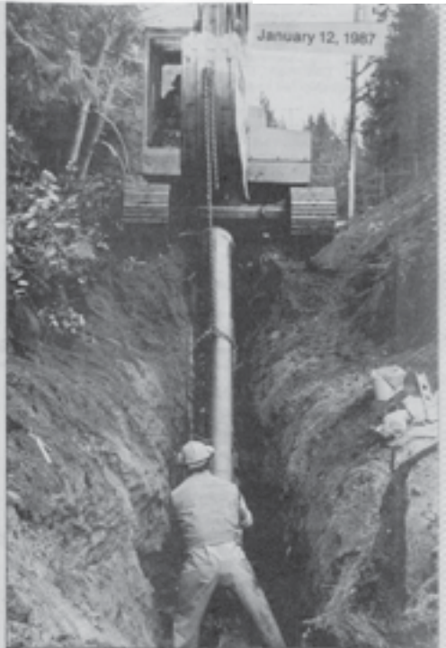
"Project #4" in the regional district's 10 Year Water Works Improvement Plan is proceeding, with 2500 metres of 14" water pipe being laid along Highway 101 from Marlene Road to Solnick's Garage. The $500,000 project requires no financing and no borrowing; it is being paid for completely from revenues.
